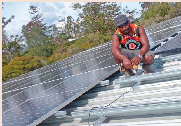
Jersey Kesa (Water and Energy Project Officer) is installing solar panels on top of the library.
